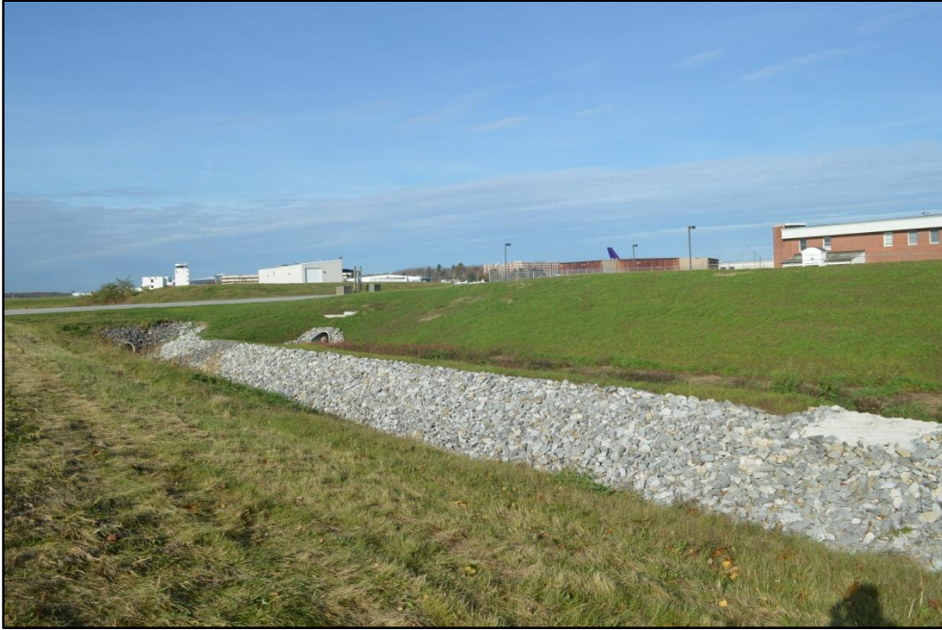
Plate 13. Large drainage swale in MU-3, view northwest, one of many such drainage features within the project limits.
