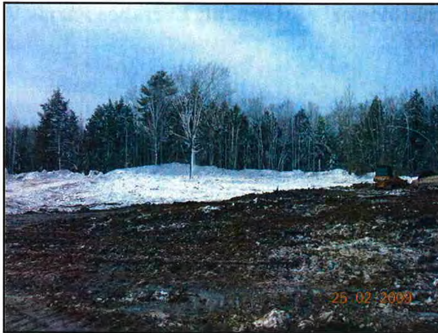
Facing southwest towards southern end of creation area - site clearing completed and initial subgrading and stump grubbing underway (Boyle Associates: February 25, 2009)
