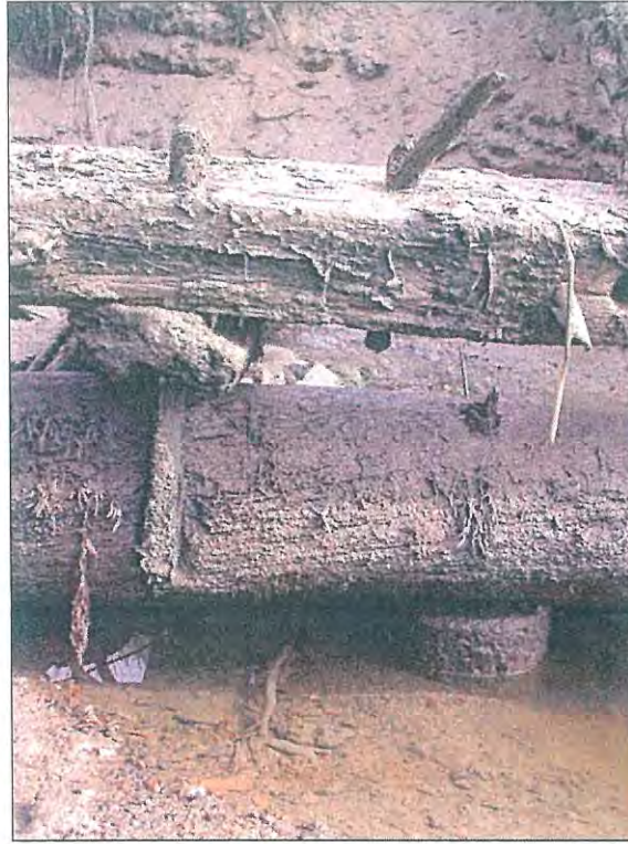
Plate 7. Wharf detail. Note the vertical pile in bottom right and treenails in upper beam.
